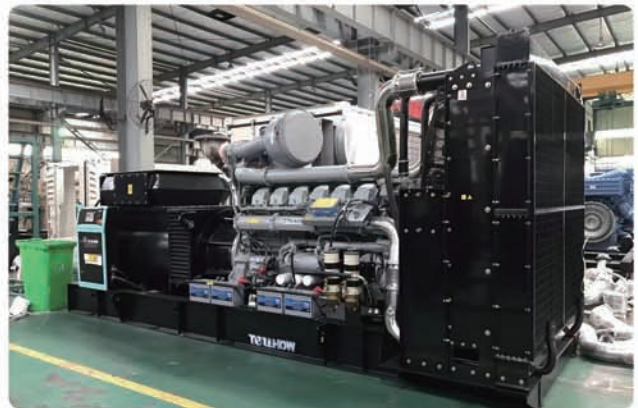
↑ Perkins Engine Radiator
